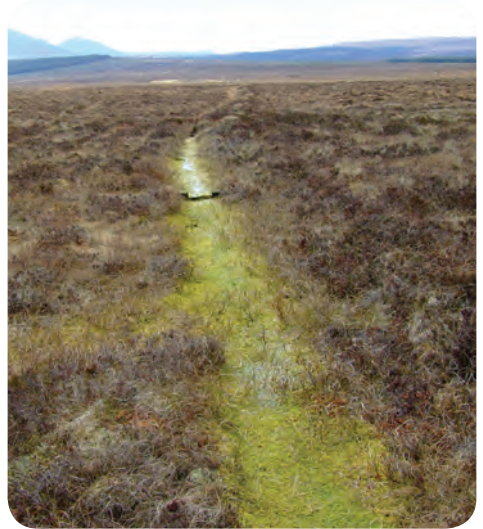
2 Drains blocked using plastic piling dams showing significant Sphagnum regrowth. Other types of peat dams can also be very effective
